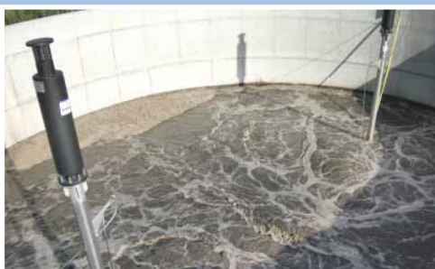
Aeratori sommersi tipo SC installati in impianto di depurazione. Submersible aerators type SC installed in a wastewater treatment plant.
